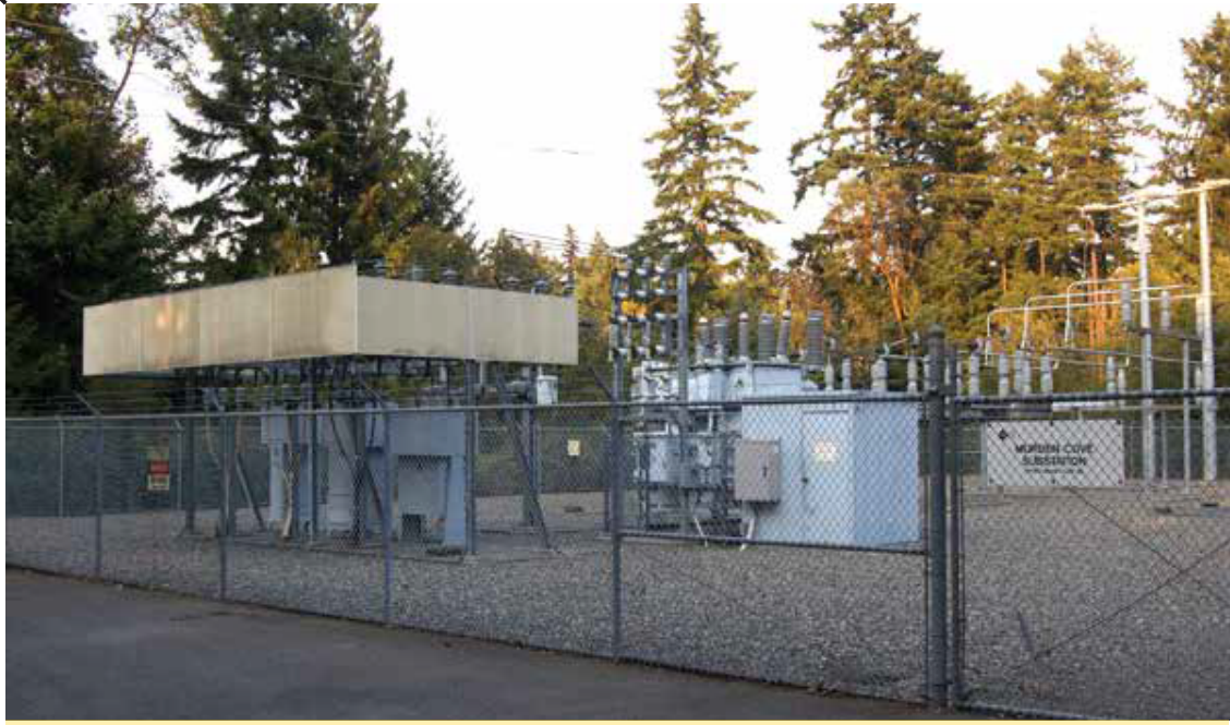
Murden Cove substation Serving 4,550 customers Originally built in 1980
