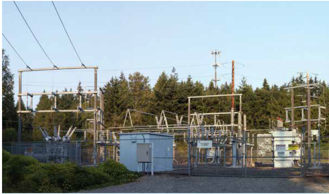
Port Madison substation Serving 4,000 customers Originally built in 1980 New transmission line and improvements in 2000
