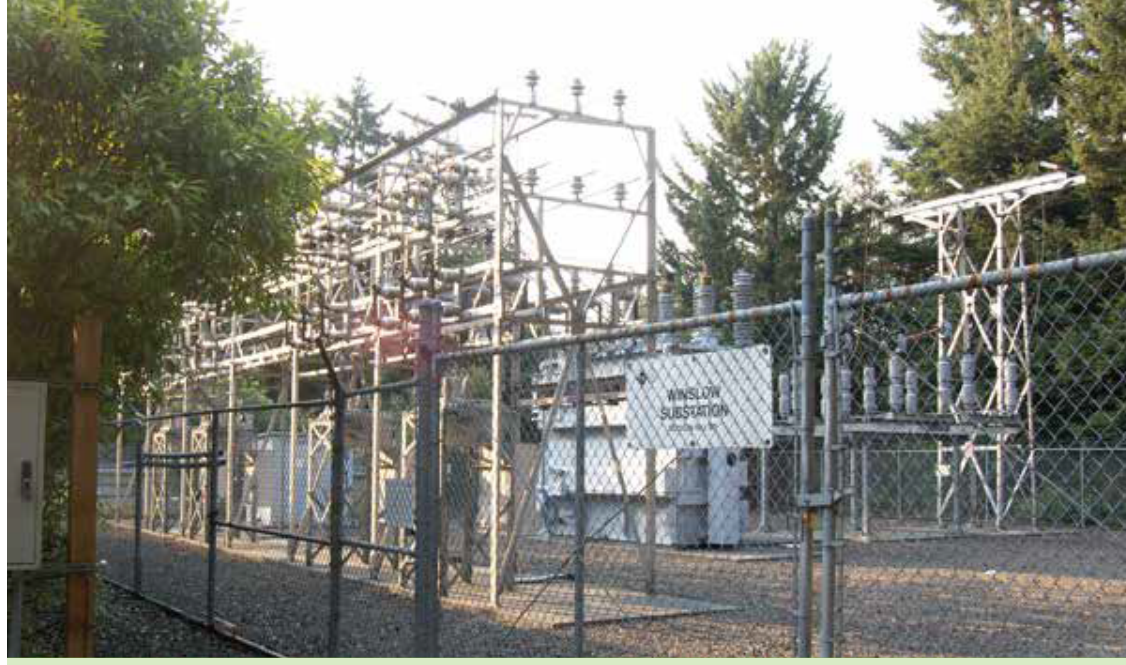
Winslow substation Serving 3,850 customers Originally built in 1960
